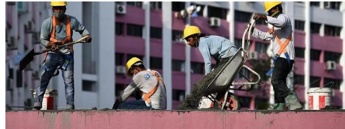
Worker who died after falling off rooftop likely disoriented from heat stress: Coroner | The Straits Times
