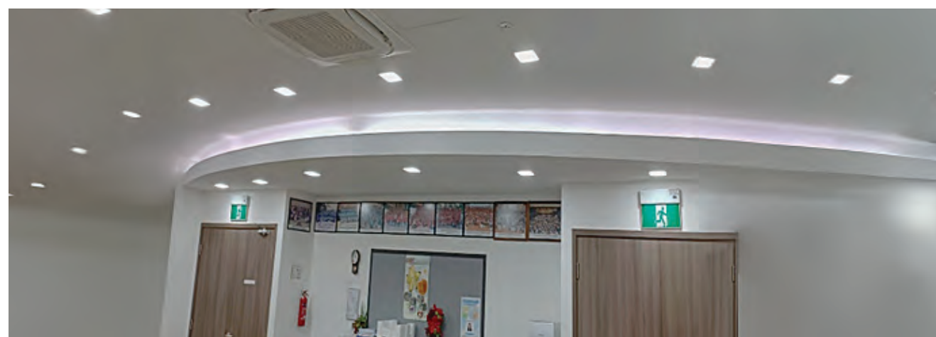
The installation of LED lights within the polyclinics under NHGP contribute to sustainable lighting.
