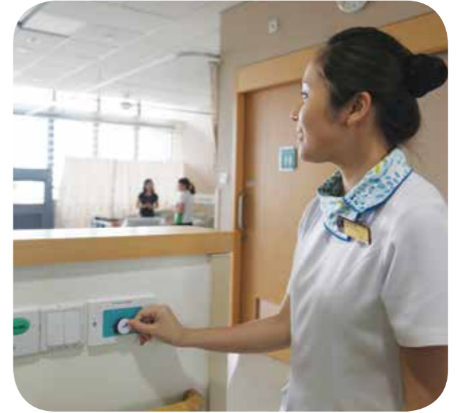
By tapping her staff pass to an RFID reader on the cubicle wall, nurses can control the opening and closing of the motorised windows in B106
