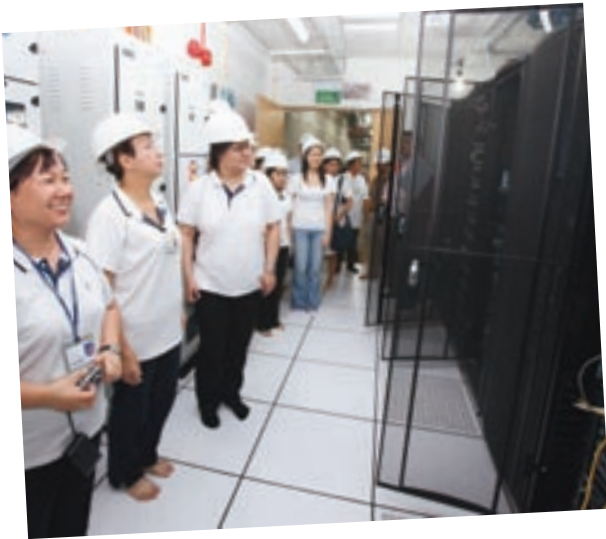
The KTPH data centre came to life on 1 October 2009
